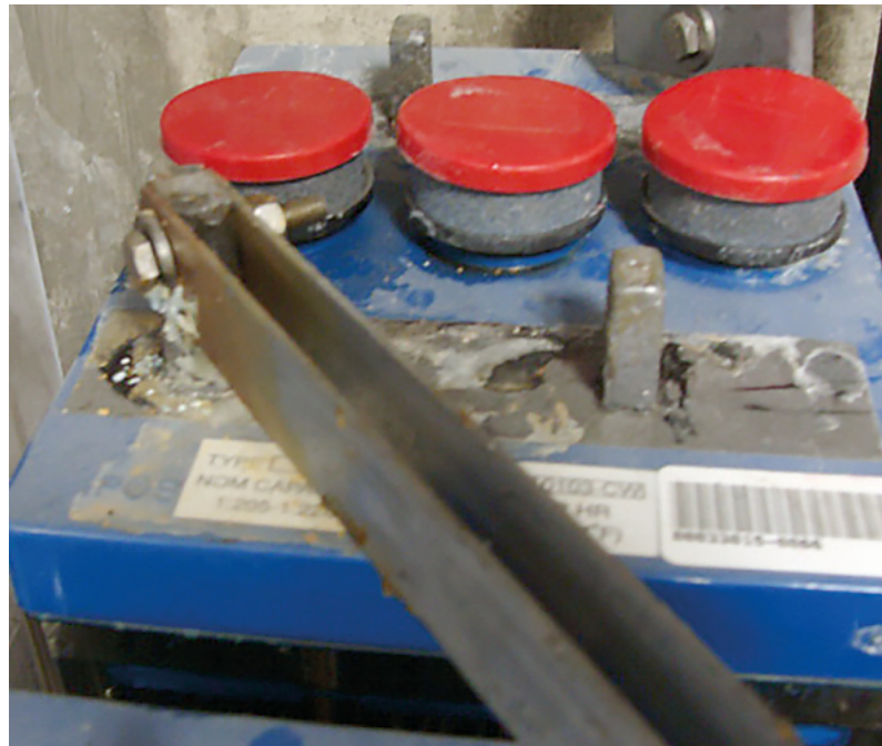
Figure 7: A typical example of poor housekeeping practice. Dust and electrolyte are present on the cell tops of this 125-volt UPS battery. The condition exists throughout the string.
