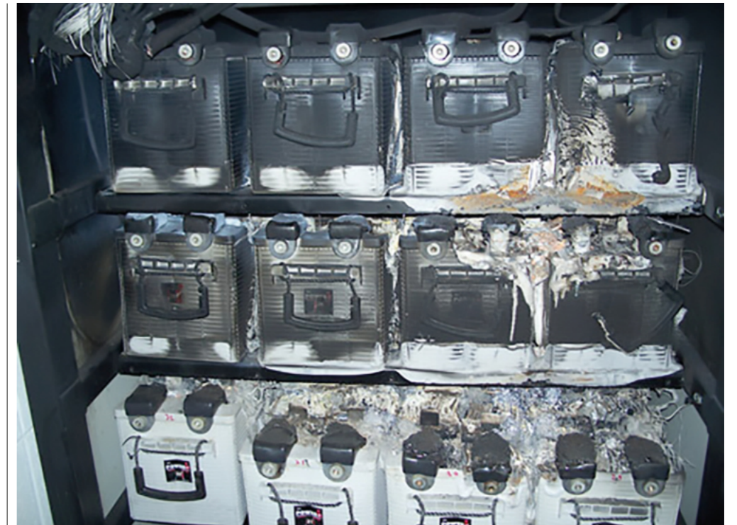
Figure 8: This photo has been widely circulated on the internet. This is clear evidence of a VRLA battery that went into thermal runaway. Such events are easily avoided by simply operating any battery per the manufacturer’s operating instructions.
